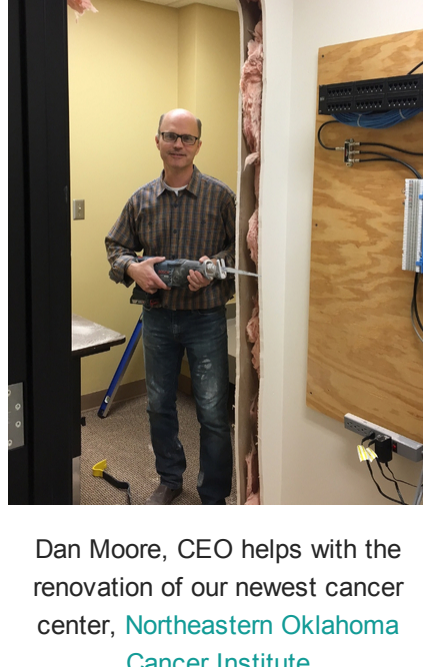
Dan Moore, CEO helps with the renovation of our newest cancer center, Northeastern Oklahoma Cancer Institute
